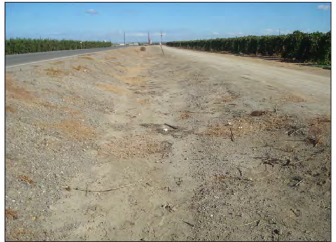
PHOTO 5: View of drainage ditch and access road along Wheeler Ridge Access Road facing north.
