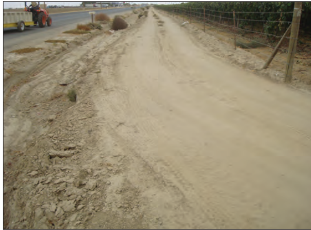
PHOTO 1: View of drainage ditch, access road and agricultural vine rows along SR-166. Photograph taken from the northwestern corner of the project site facing east.
